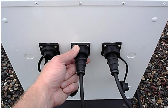
Figure 18 Connect Solar Panels to Battery Enclosure Box
