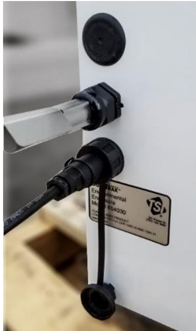
Figure 28: Power Cord from Solar Battery to Environmental Enclosure
