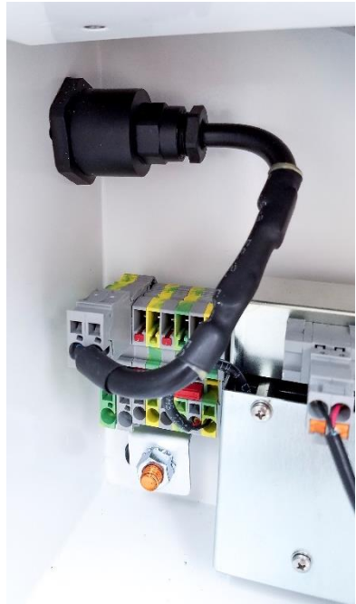
Figure 27: DC Cable to DIN Rail
