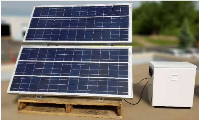
Figure 26: Solar Cell Power System
